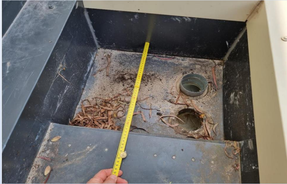
Non-compliant sump with an inverted pop used as a standing overflow pipe
