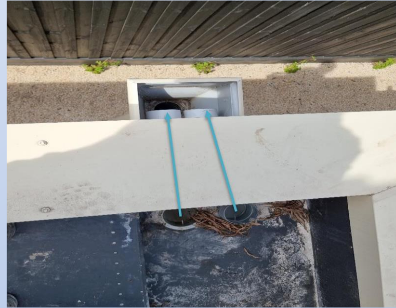
Both the primary and overflow pipes discharge into a rainhead – non-compliant (the overflow must discharge visibly to atmosphere and the surface drainage system)
